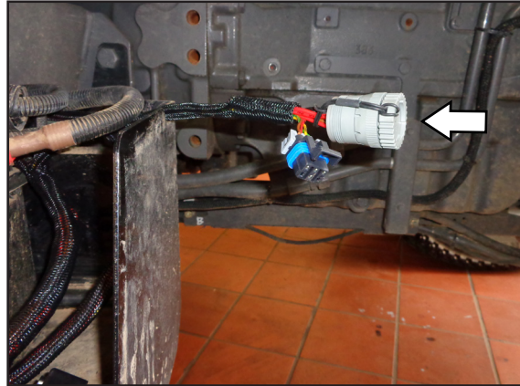
Fig. 57: X05A and X04A terminal of the main harness
